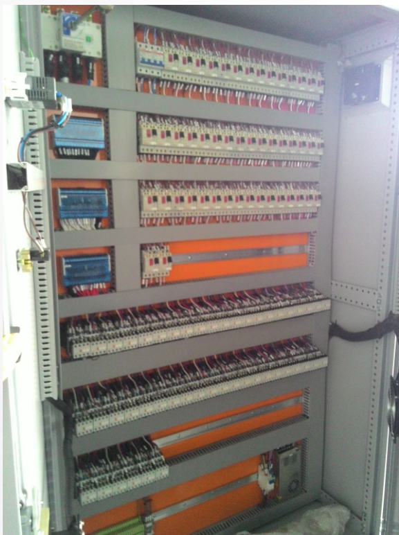
Painél de comando interior
